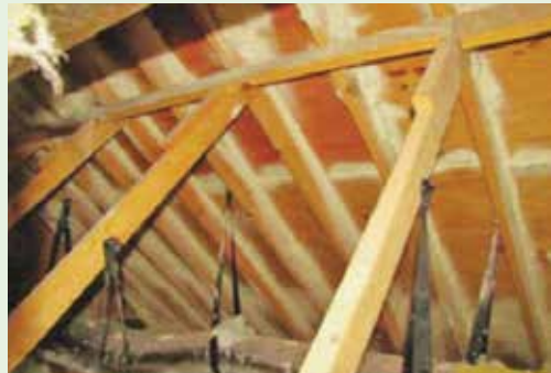
Figure 5-5. Spray polyurethane foam is used to add strength between the rafters and the plywood sheathing. This method can be used to strengthen existing roofs and may negate the need to replace older roofs. It can also be used where fasteners are missing or at the corners of hip style roofs or the ends of gable end roofs, which are especially susceptible to wind forces. See FEMA publication numbers P-499 and P-804. Image courtesy of FEMA
