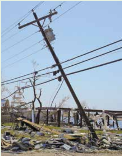
Figure 5-25. Downed or damaged power lines in a residential area can pose a serious danger to public safety. Image courtesy of U.S. EPA
